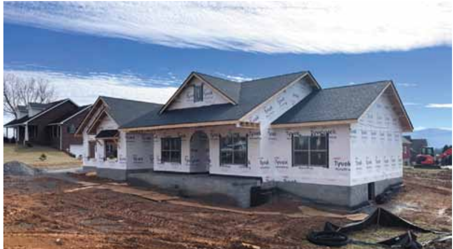
A new home under construction by Idell Construction in the Long View subdivision.
