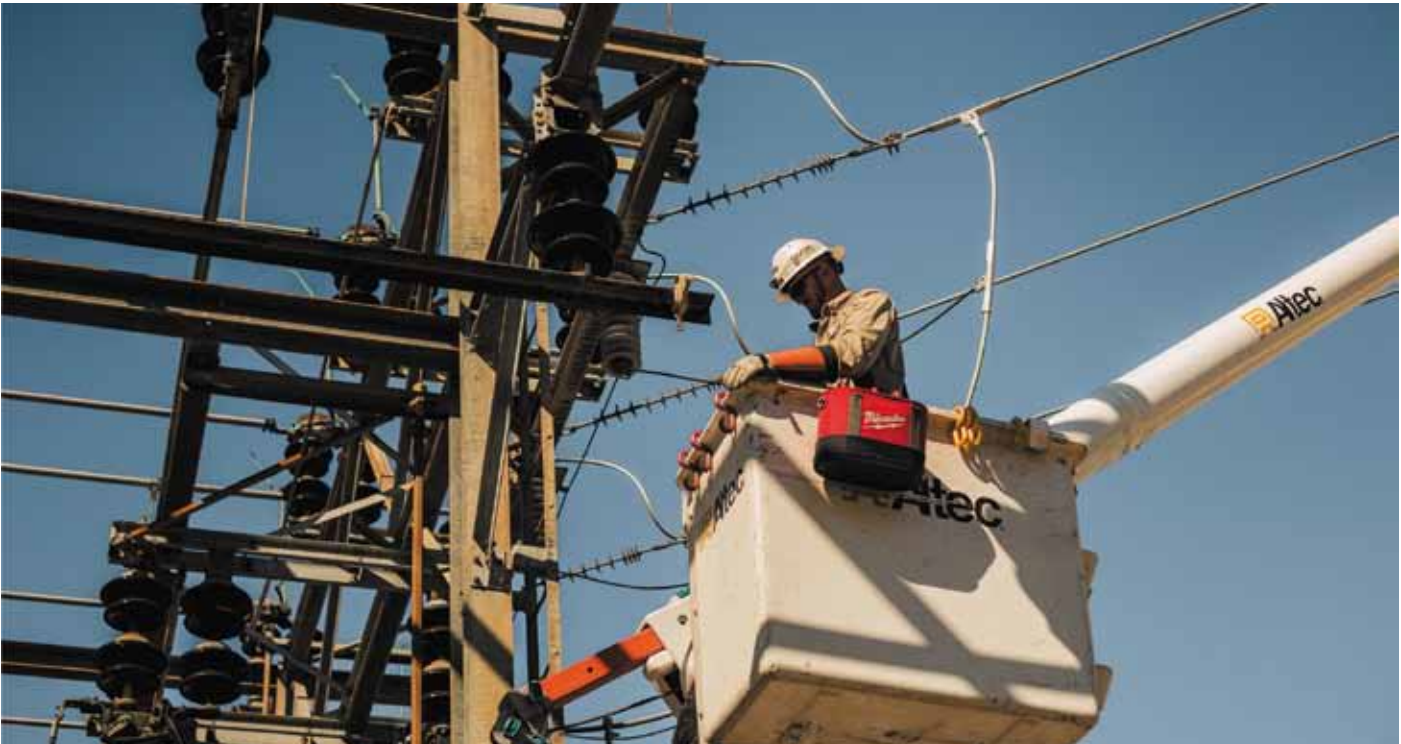
A GEA lineman in action, high above in a bucket truck, fine-tuning a substation ensuring seamless operation.
