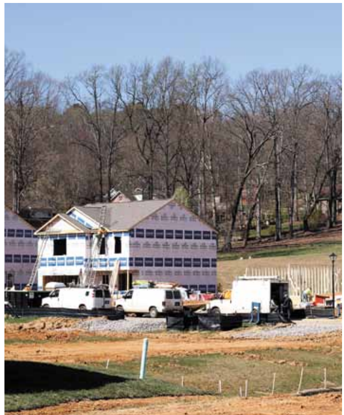
Crews work on framing homes located in the Wildwood Landing subdivision which features 31 single family homes.
